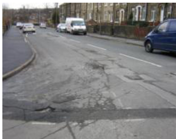
Potholes, image courtesy of David Mazurke
