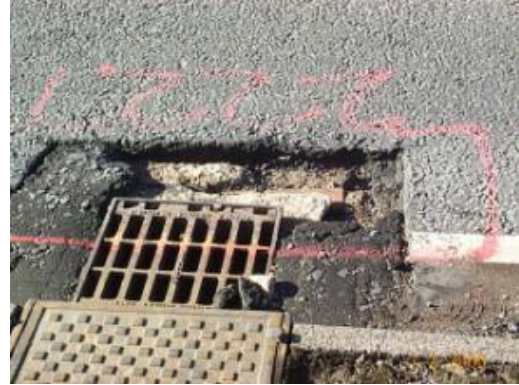
Damage to ironworks, image courtesy of Atkins
